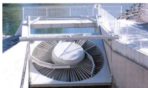
Photo 17 : Turbine VLH (source : MJ2 Technologies)
